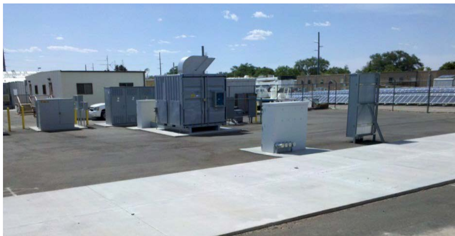
Figure F-3. Energy Storage Test Pad at Sandia National Laboratories, Albuquerque, NM
