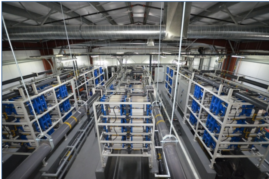
Figure 46. Prudent Energy 600-kW/3,600-kWh VRB-ESS Installed at Gills Onions, Oxnard, CA
