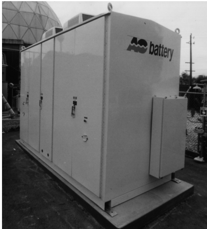
Figure 123. First AC Battery PM250 modular battery system installed at Pacific Gas & Electric's Modular Generation Test Facility, San Ramon, CA, in 1993.
