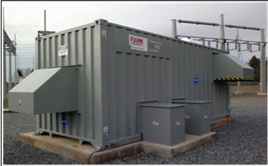
Figure 39. FIAMM 222-kWh System Site at the Duke Energy Rankin Substation
