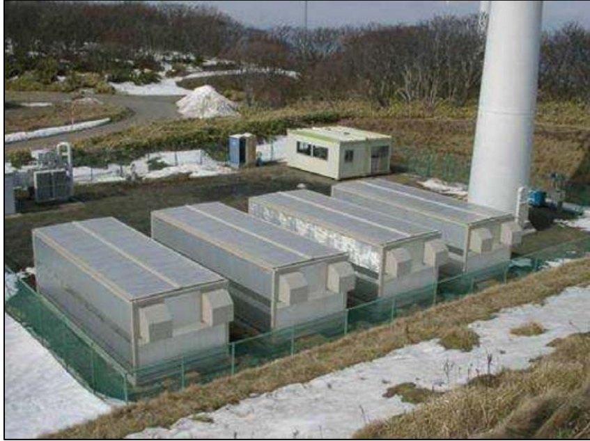
Figure 71. Acid Battery Installation at Tappi Wind Park (Courtesy Hitachi) 49
