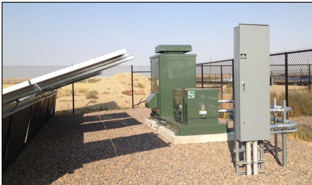
Figure 40. Containerized 25 kW/50 kWh FIAMM Battery Unit (large green housing) on Concrete Pad, Next to S&C PureWave CES (small green housing)
