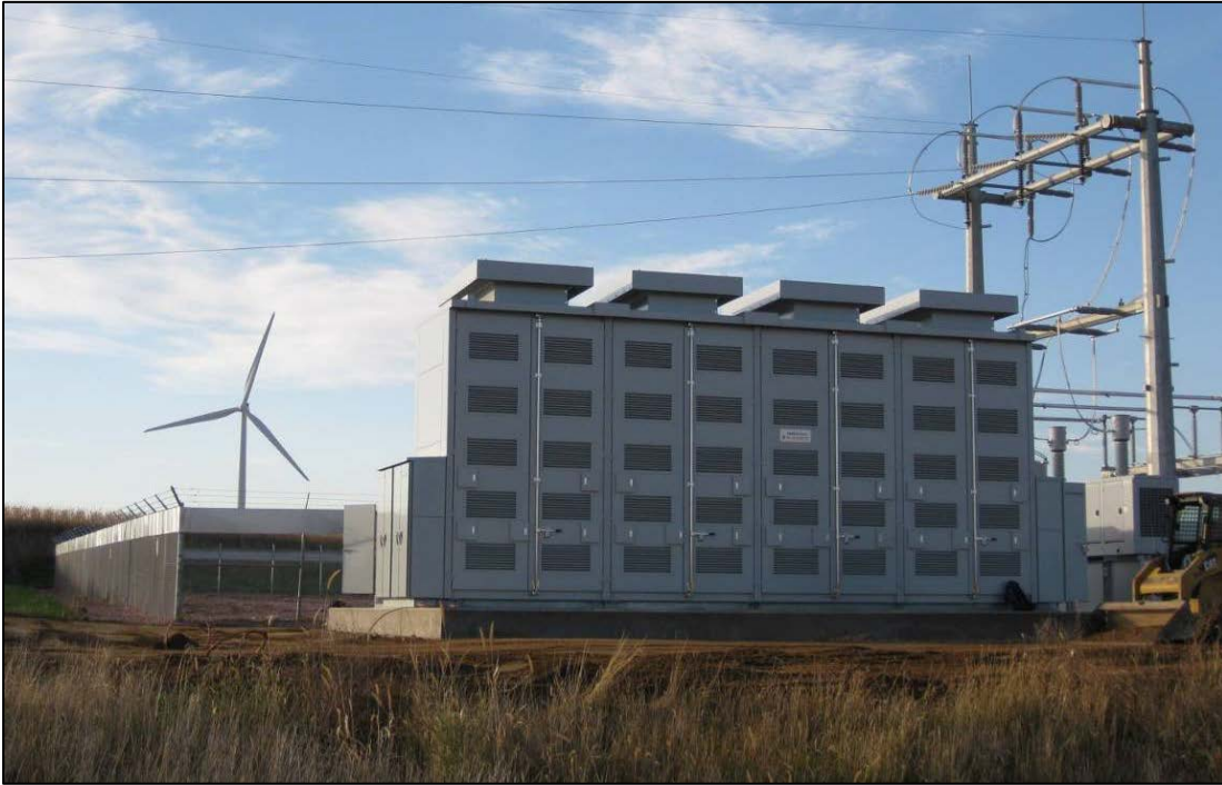
Figure 34. Xcel Battery Supplementing Wind Turbines, Lucerne, MN
