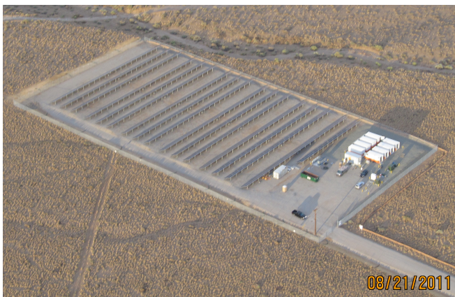
Fig. 1. Aerial view of the 0.5 MW Prosperity PV plant with battery storage. The plant occupies approximately four acres (16,000 m 2 ). The shifting and smoothing batteries are in the white containers.
