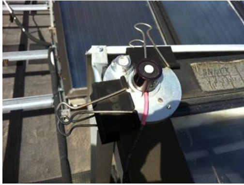
Figure 5-15. Externally Mounted Li-Cor global irradiance sensor.
