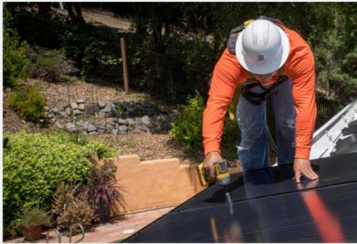
Installers add solar panels to a residential roof in Lafayette, Calif. Photographer: David Paul Morris/Bloomberg via Getty Images
