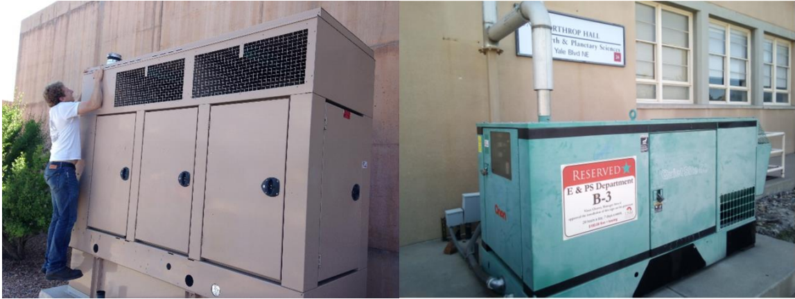
Figure 2-6. Distributed Generation Resources at UNM; Left: 150 KVA diesel generator with author for scale, located at the Architecture building at UNM; Right: 50 KVA generator at Northrop Hall UNM.
