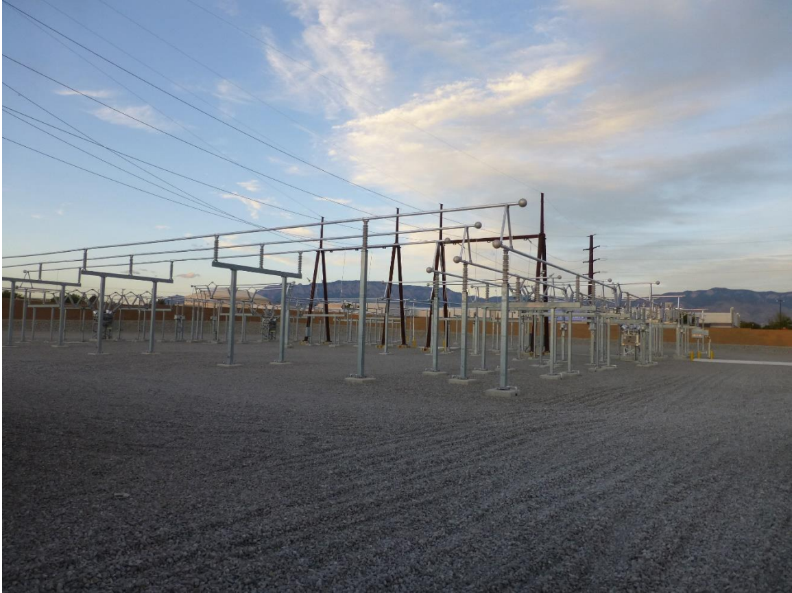
Figure 2-3. Richmond Switching Station in Albuquerque, NM; similar in function and size to a utility scale Point of Common Coupling (PCC).
