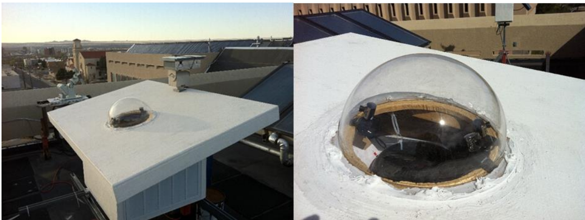
Figure 5-14. External Enclosure with the clear dome.
